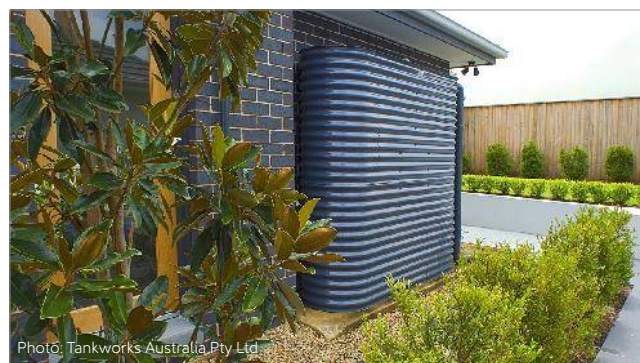
Slimline tanks installed along a wall save space while saving water.
